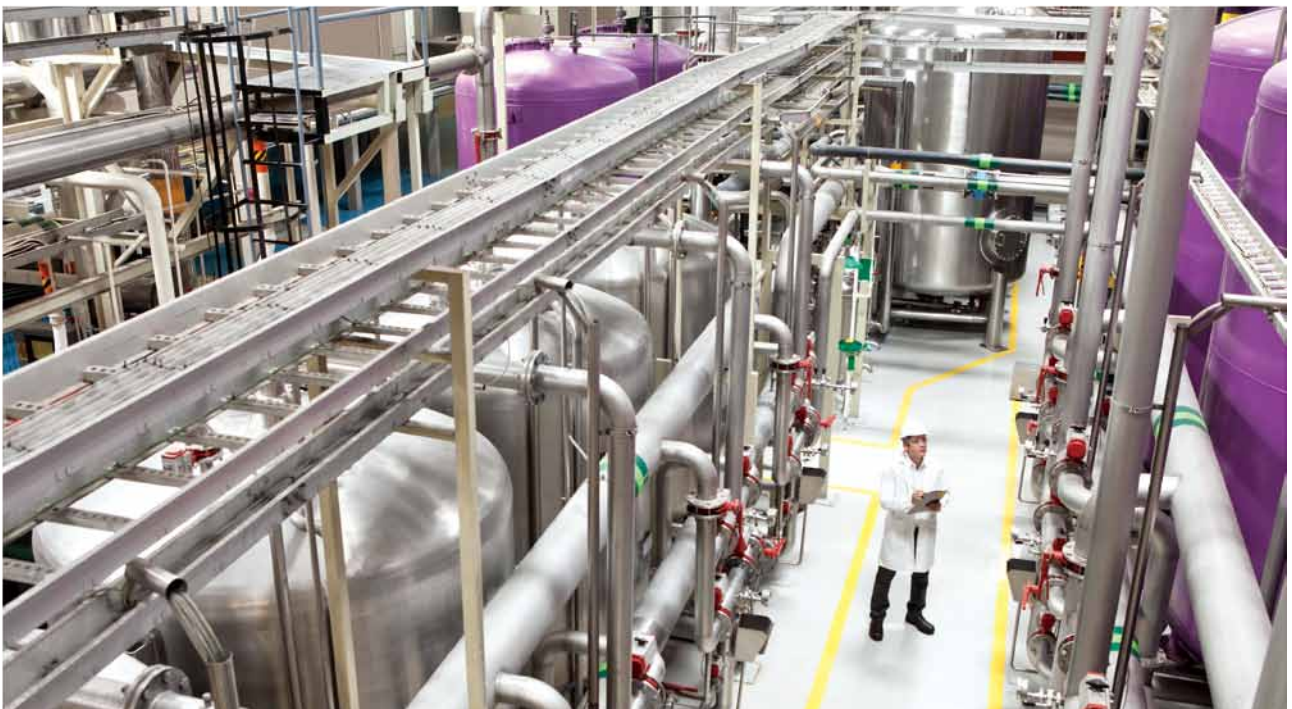
Figure 1. Gaining access to field devices plays a pivotal role in securing productivity and smoothing plant operation.
